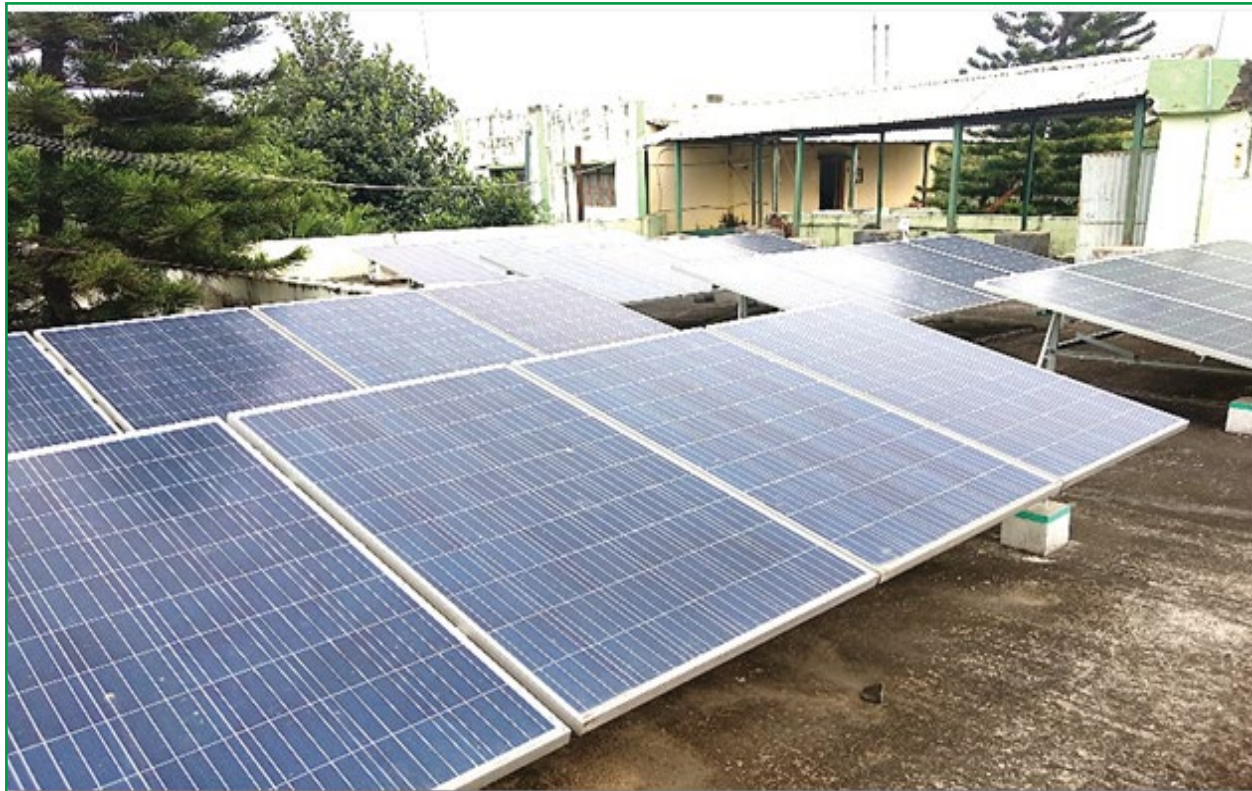
35 KWp Roof Top Solar Panel, Jhanjra
