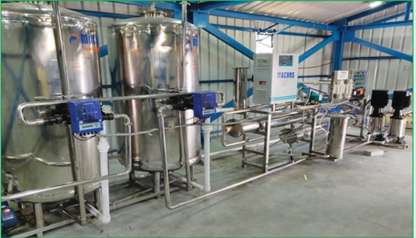
RO Water Treatment Plant, Satgram (capacity 5000 L/Hour)
