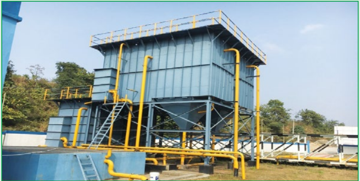
Dalmia Water Treatment Plant (2.5 LCuM/year)
