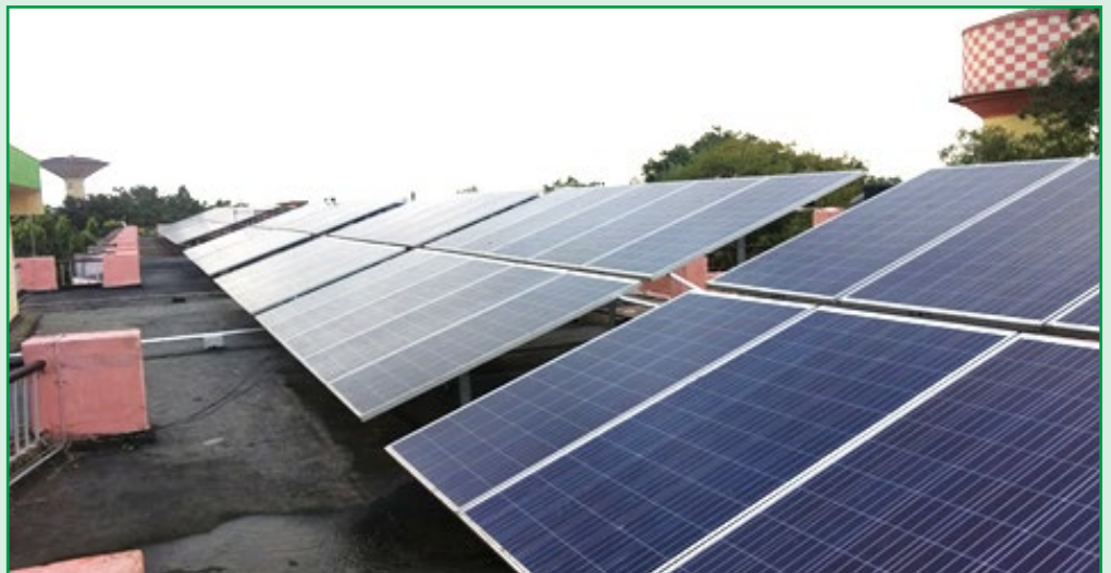
30 KWp Roof Top Solar Panel, Bankola
