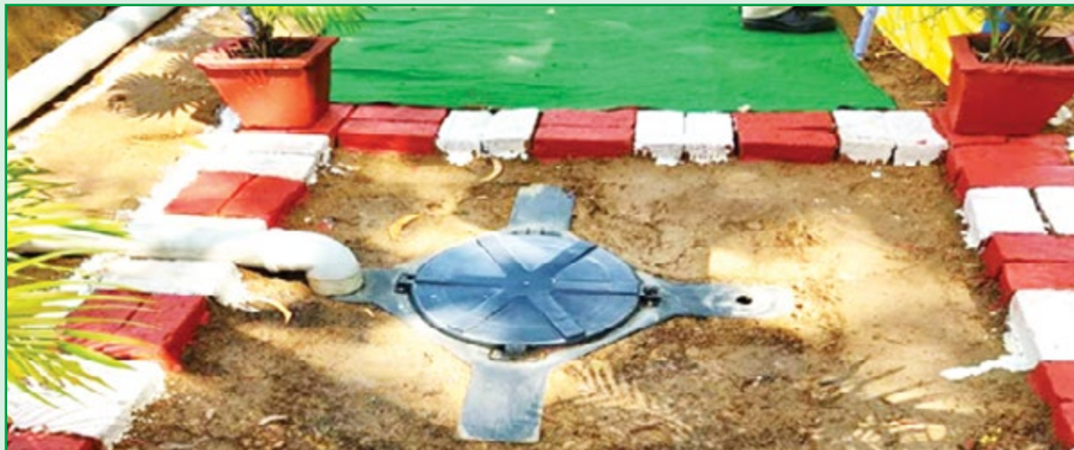
Rain Water Harvesting Plant, Sonepur Bazari Catchment Area 3000 sqft
