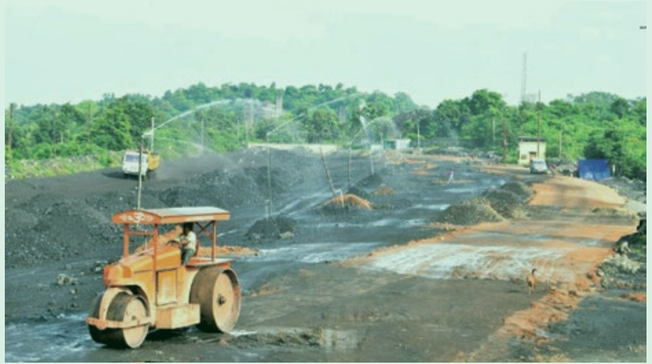
Fixed Water Sprinkler, Bonjemehari
