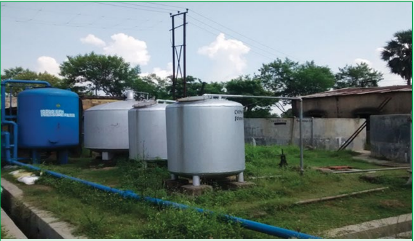
Pressure Filter Plant, Jhanjra (Capacity 32000 GPH)
