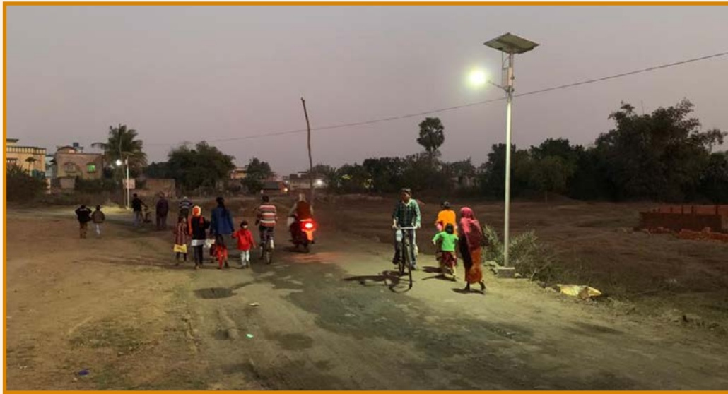
Solar Street Lights at village road
