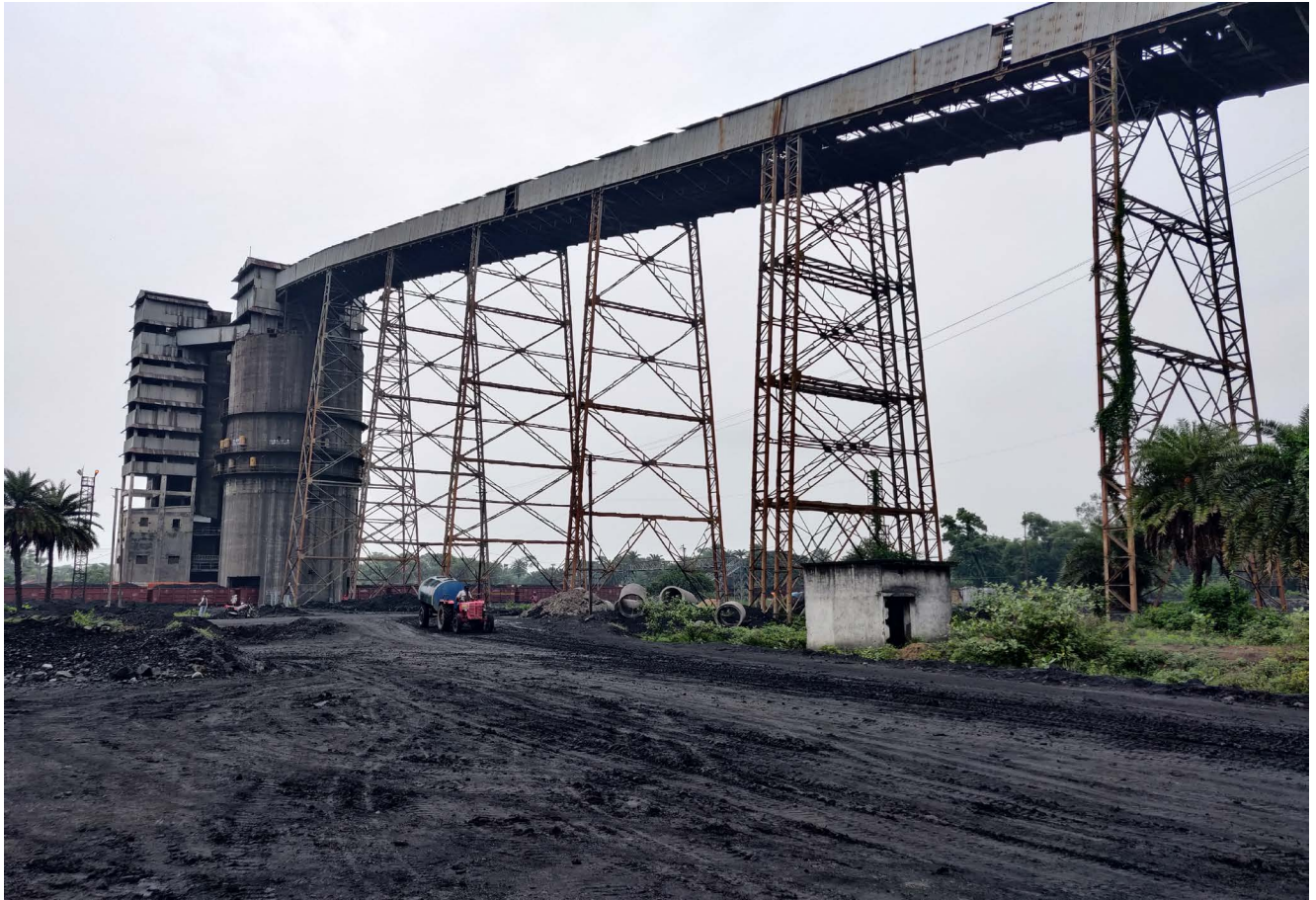
CHP at Rajmahal Area
