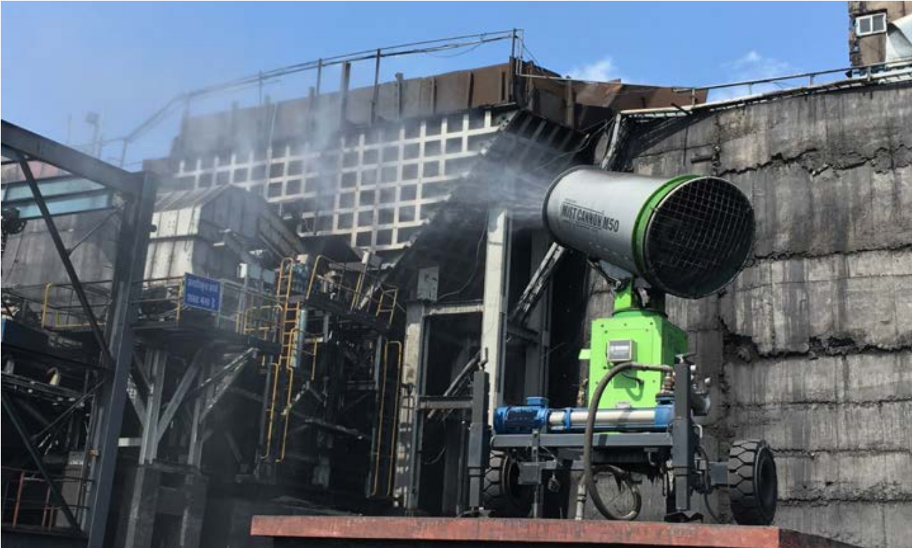
Mist Gun for effective dust suppression at CHP
