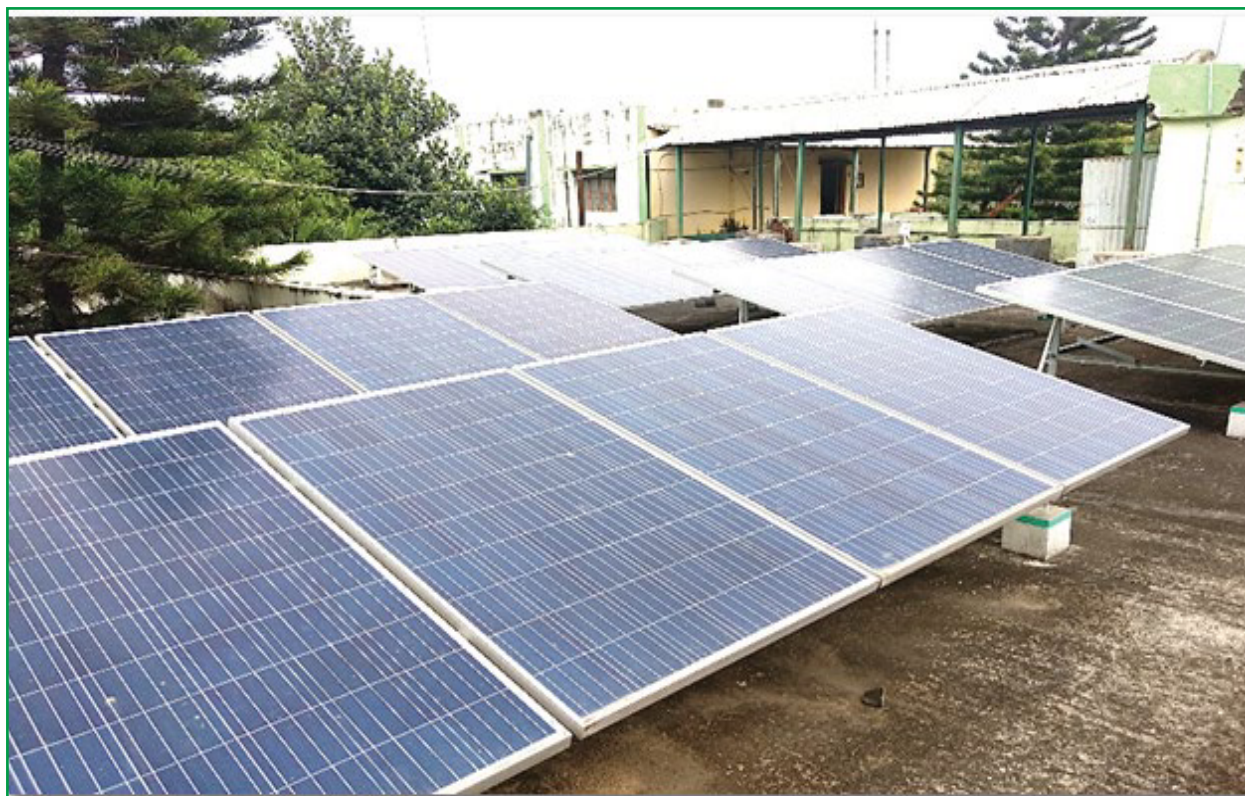
35 KWp Roof Top Solar Panel, Jhanjra
